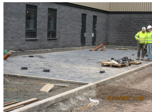
Block paving for disabled person parking bays being installed on the East elevation
